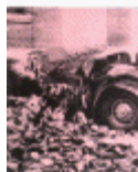
(Bottom) Long Beach, California, 1933. Exterior walls collapsed onto parked cars after this magnitude 6.3 earthquake (photo by Southern California Earthquake Pictures).
